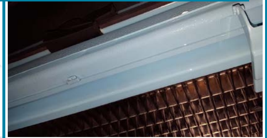
PHOTOS OF ICE MACHINE 30 DAYS AFTER INSTALLING SANIT-ICE
